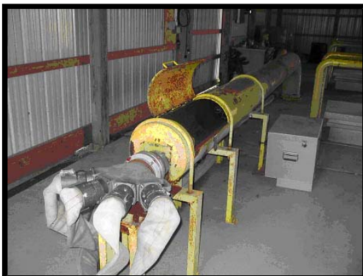
Photo 3: The test re-entry port is designed to direct the water to the far end of the baffled, underground tank.
