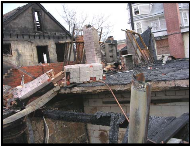
This is what the Charlie side looked like when it was all said and done.
